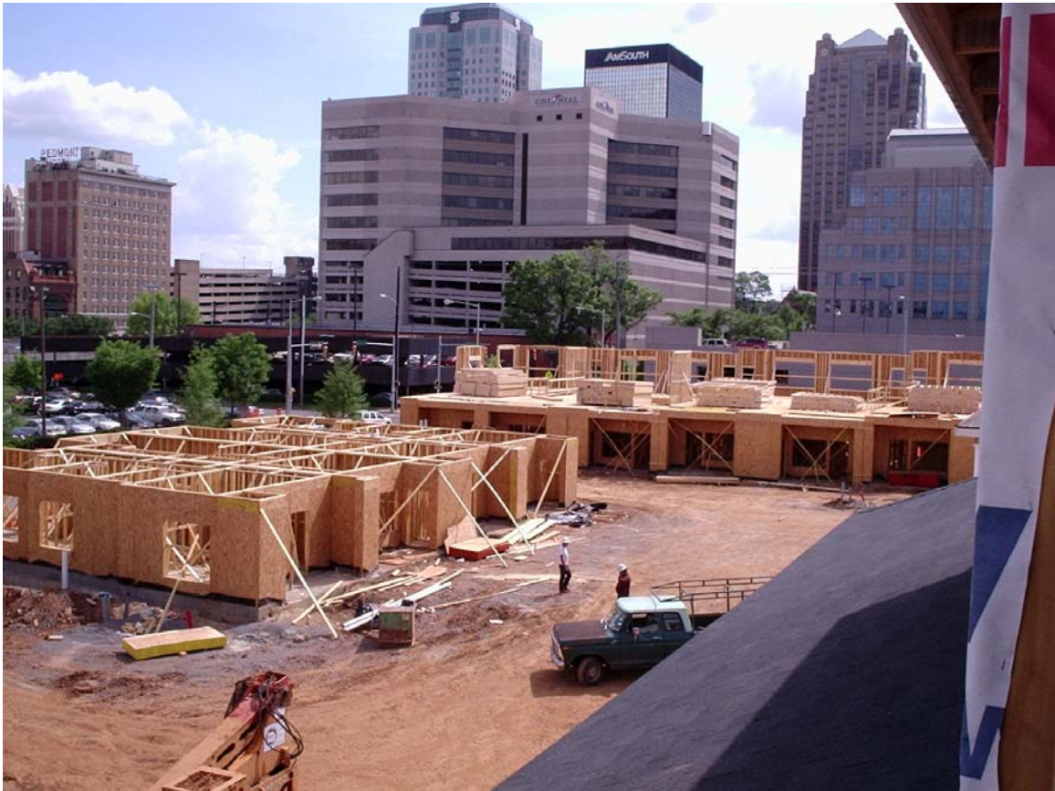
BLOCK 'B' - BUILDING'S 16 & 17 From The 3 rd Floor Of Building 14 – A View Of Downtown
