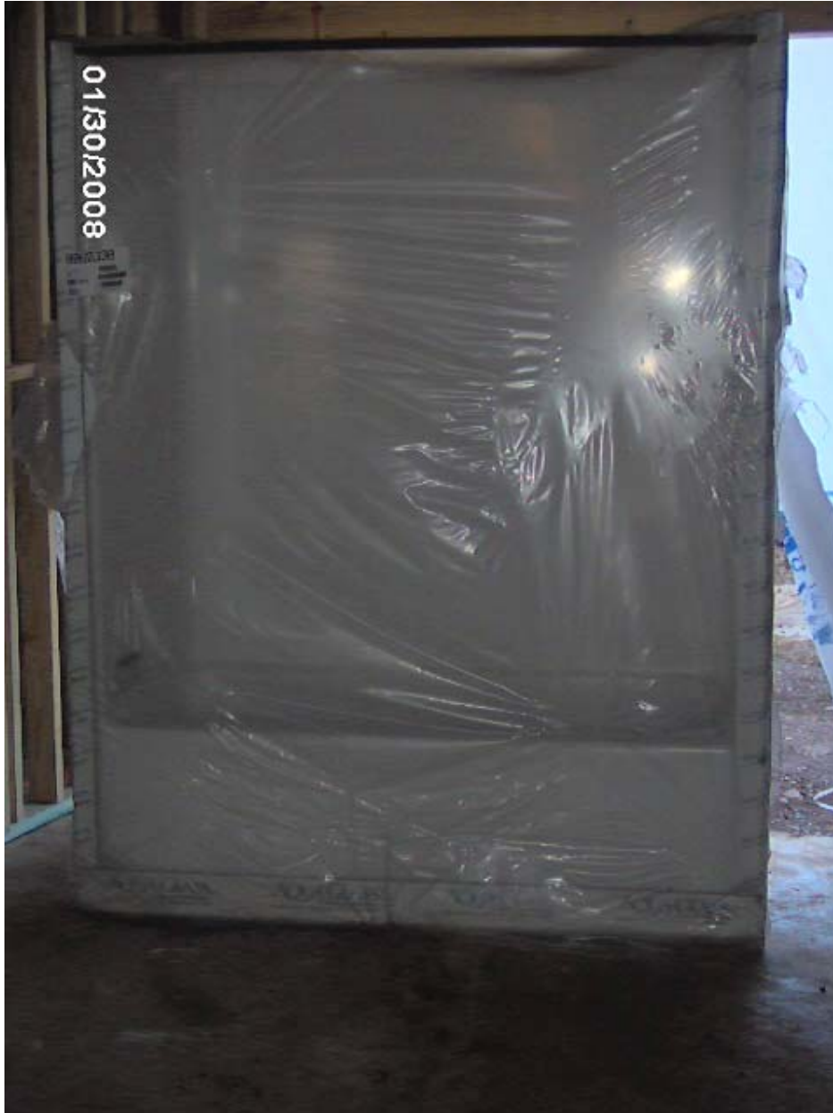
PARK PLACE - PHASE III Tub/Shower Fixture in Protective Wrapping, Prior to Installation
