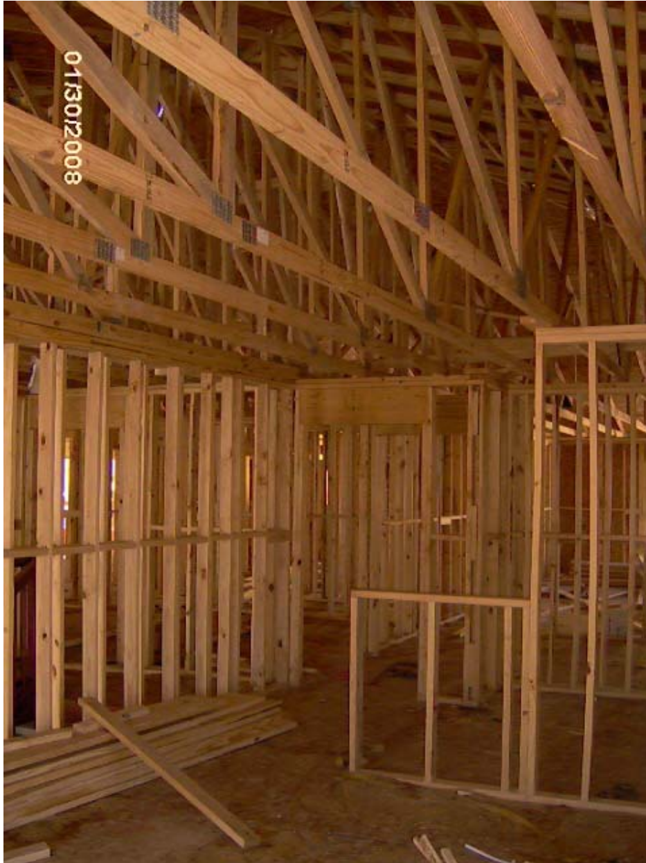
PARK PLACE - PHASE III Upper Level Interior Partition Framing with Roof Truss Above
