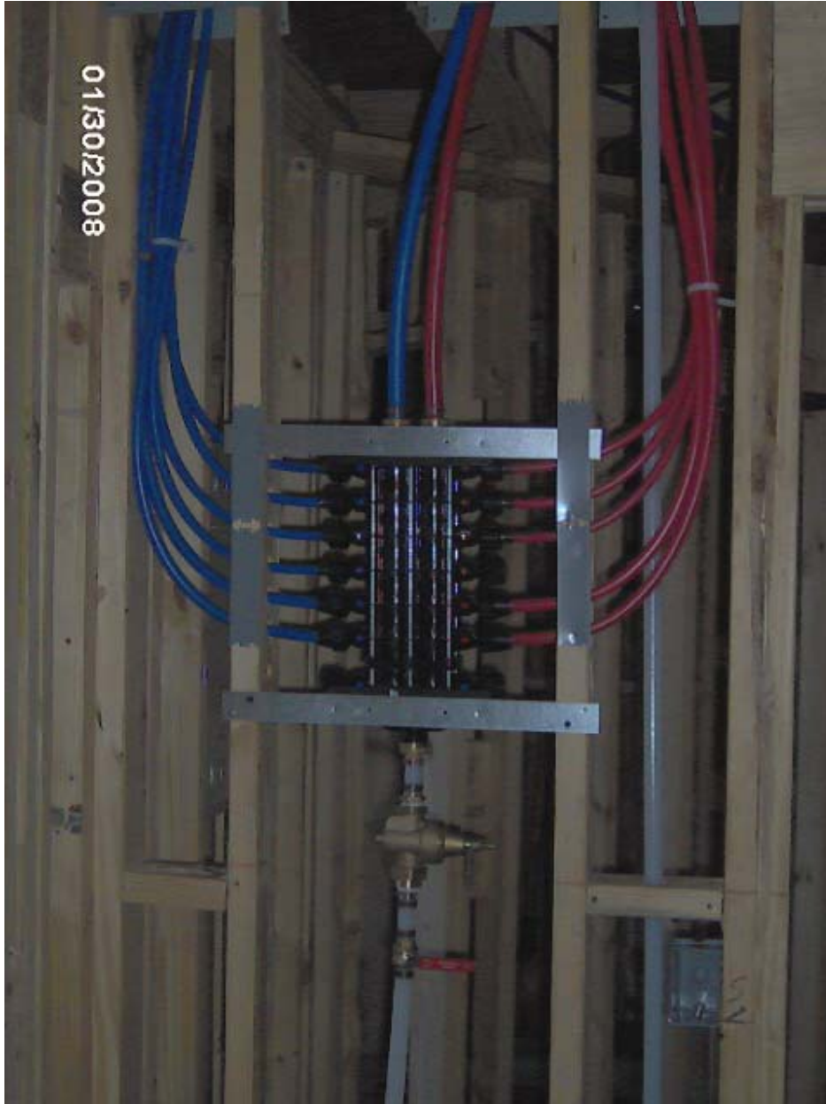
PARK PLACE - PHASE III Interior Plumbing Distribution Panel
