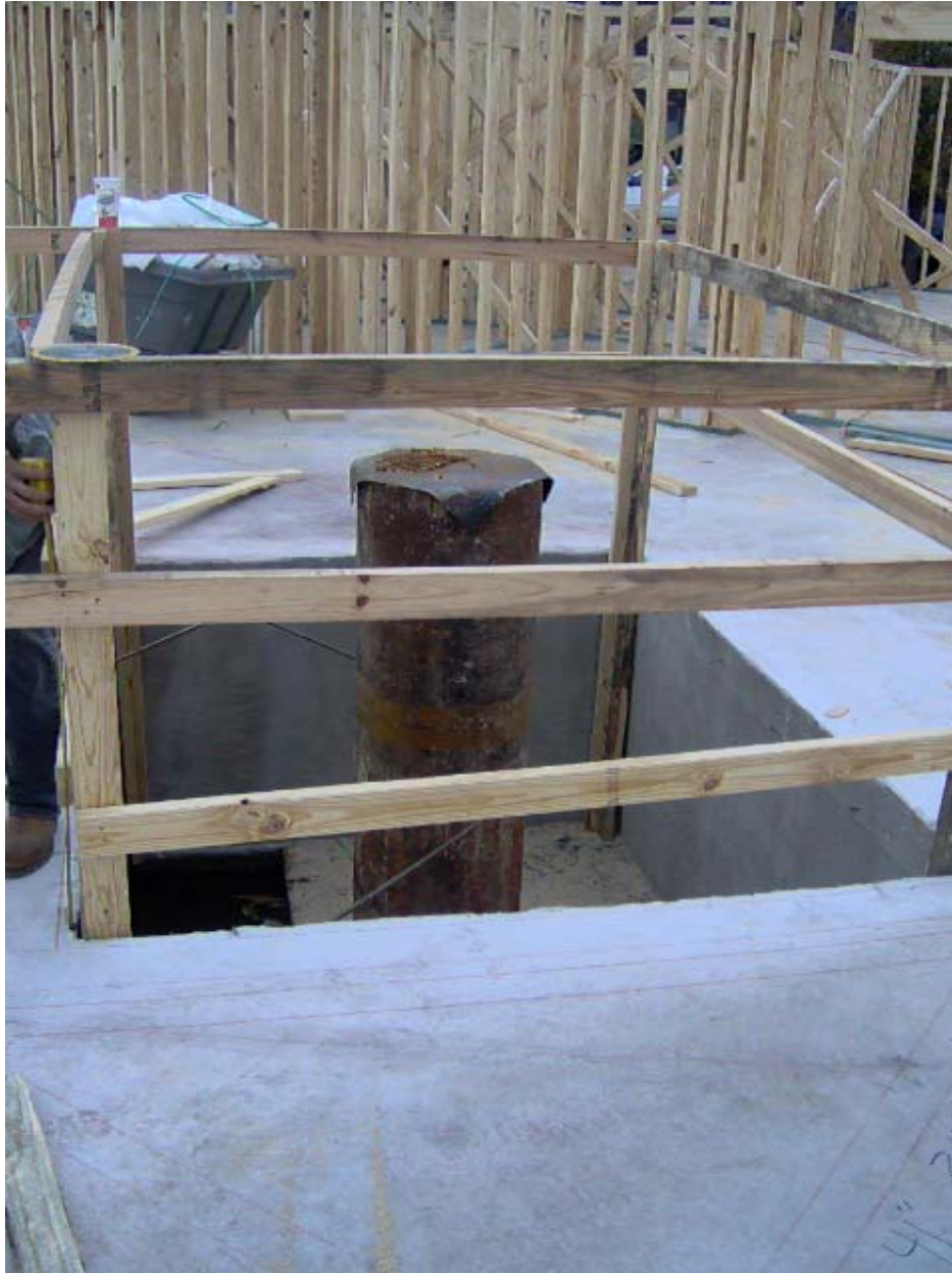
PARK PLACE - PHASE III Elevator Pit/Plunger
