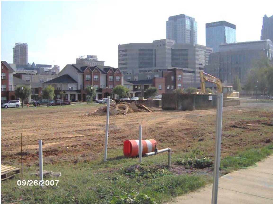
PARK PLACE - BLOCK 'B' NORTH Site Clearing/Cleaning in Prep for Construction of Mid-Rise Building
