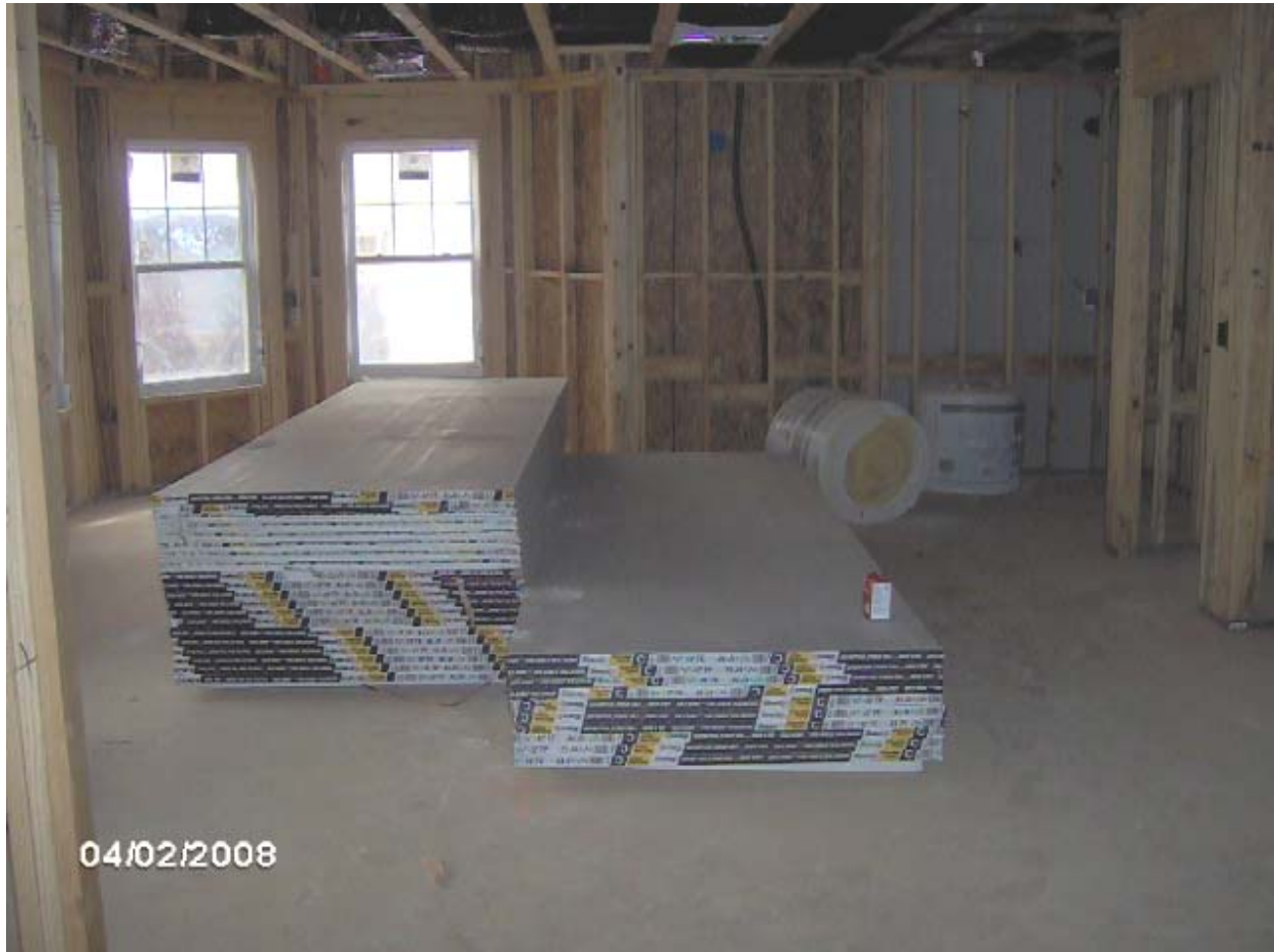
PARK PLACE - PHASE III Stockpiled Gypsum Board on an Upper Level
