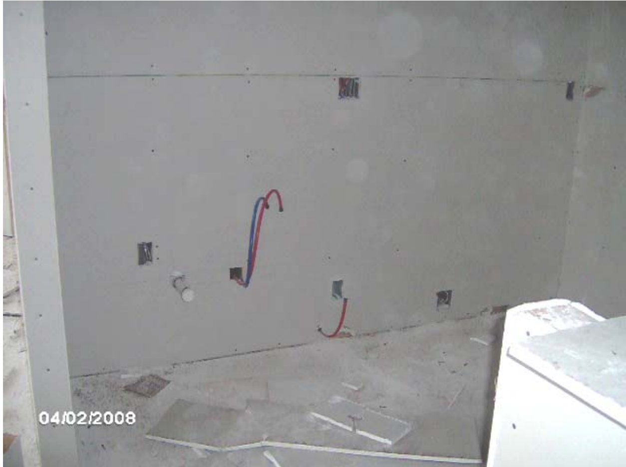
PARK PLACE - PHASE III Kitchen Plumbing Wall
